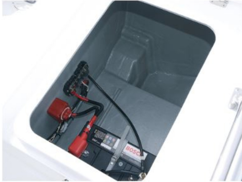
Port stern locker (battery space)
